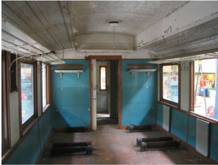
This photograph shows the situation before the work inside started. Here is the part of the coach that later became the bar counter
